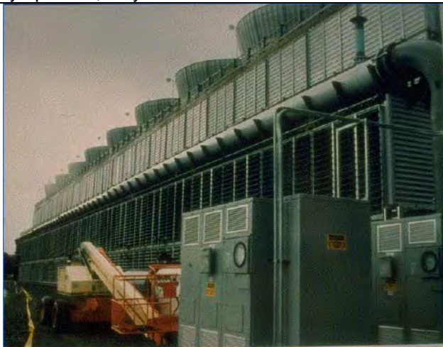
Operational plume-abated tower, ~60 ft. tall – Selkirk 2 Cogen, 330 MW (NY) Source: P. Lindahl – Marley presentation, May 2002.
