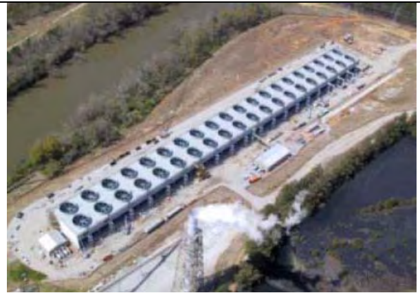
Retrofit 40-cell back-to-back inline conventional cooling tower, coal-fired Plant Yates (GA) – 40 cells is adequate size for up to 1,100 MW nuclear reactor.
